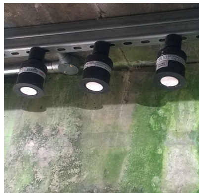
3 dBi HART transducers Monitoring Sluice Levels
